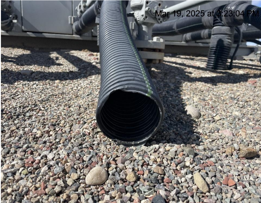
Photo # 5397 Flowline heating insulation open ended /wildlife hazard/available for entry by wildlife
