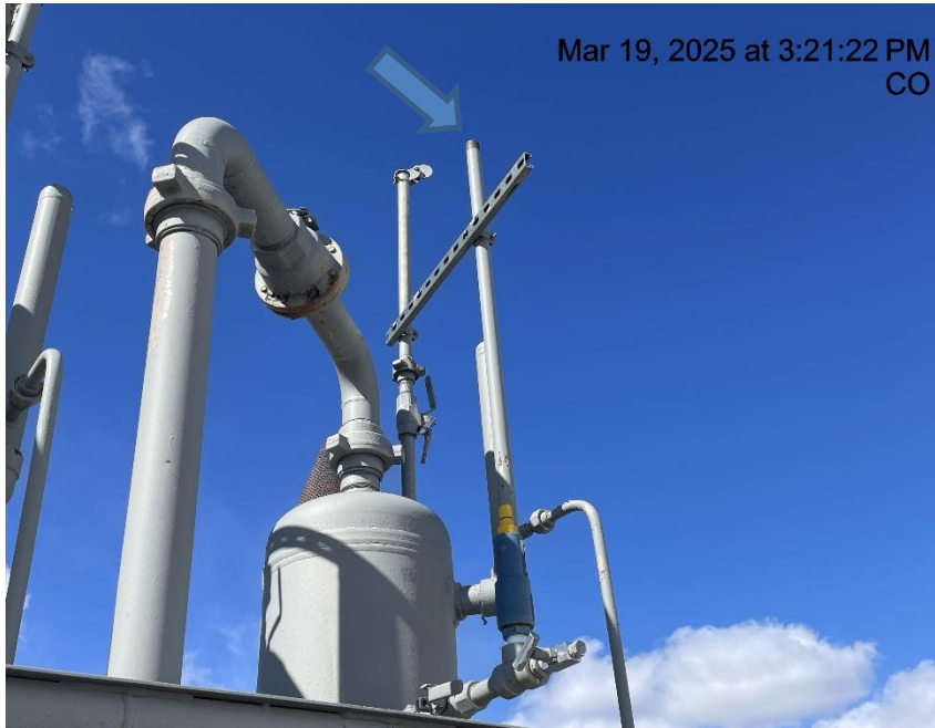
Photo # 5393 PRV vent line does not comply with CECMC pressure safety device rules
