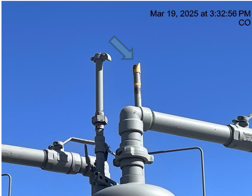
Photo # 5395 PRV vent line does not comply with CECMC pressure safety device rules
