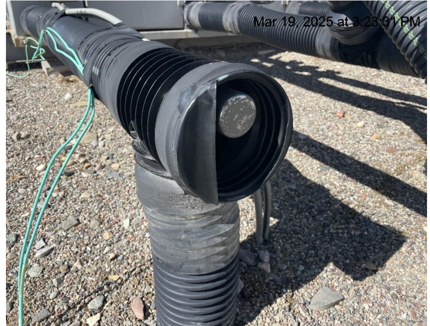
Photo # 5392 Flowline heating insulation open ended /wildlife hazard/available for entry by wildlife
