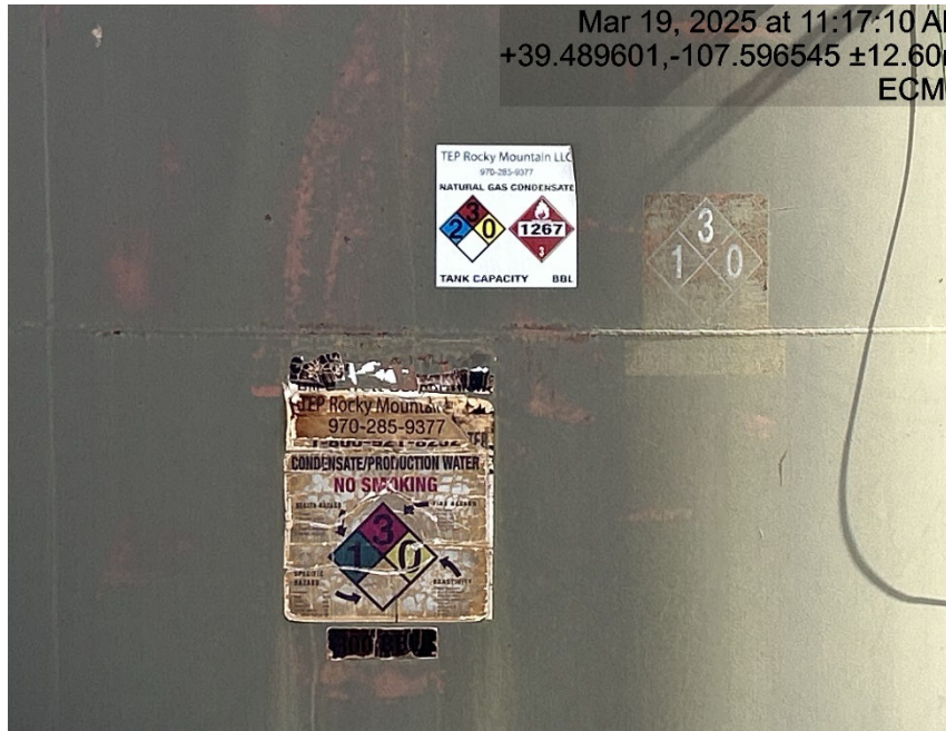
Labeling lacking information (quantity)
