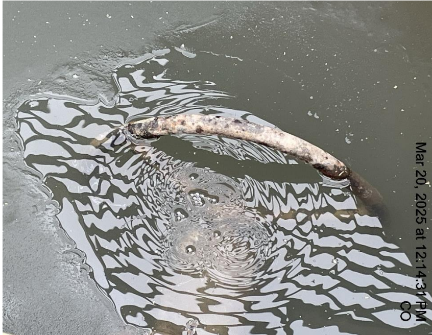
Photo # 5667 Mechanical Condition - Possible leak on CSF 42B-07-07-91 wellhead casing valve
