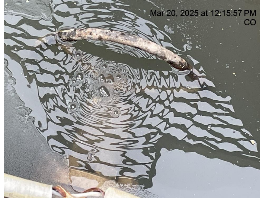
Photo # 5668 Mechanical Condition - Possible leak on CSF 42B-07-07-91 wellhead casing valve
