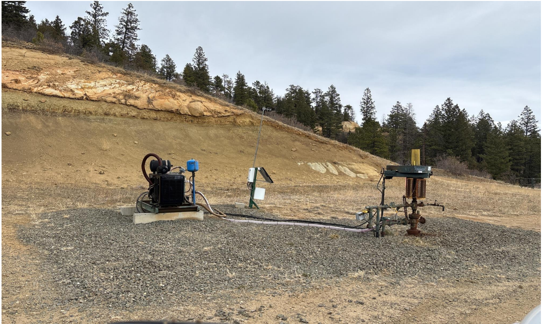
PHOTO 3: WELLHEAD AND EQUIPMENT.
