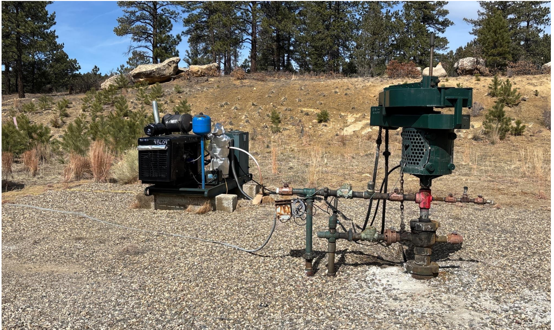
PHOTO 3: WELLHEAD AND EQUIPMENT.
