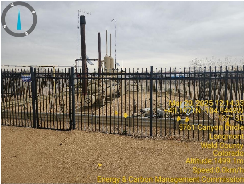
Photo 3 Horizontal heated separator.
