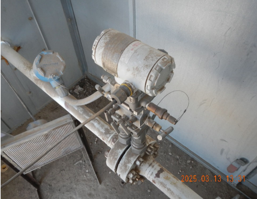
3. Gas meter inside meter shed.
