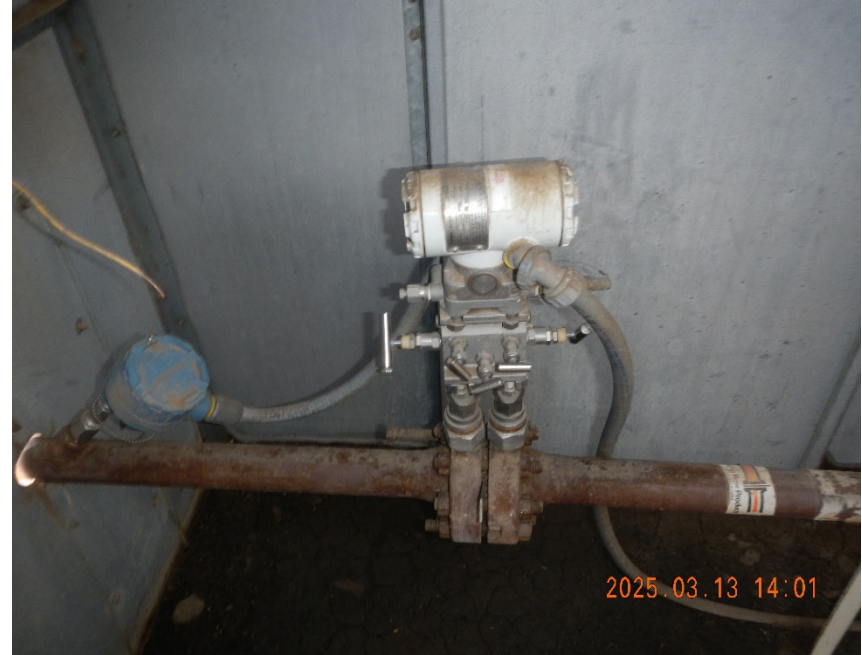
6. Gas meter inside meter shed.
