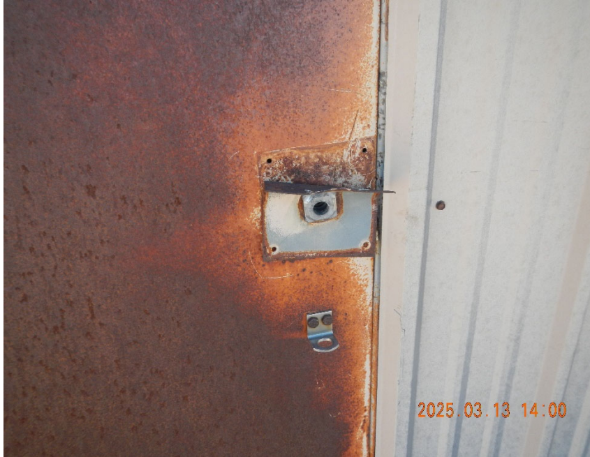
5. Damaged shed door with missing handle. Door is jammed and inspector unable to access.
