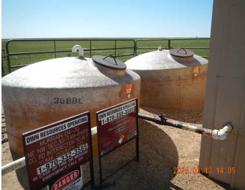
7. Produced water tanks (30 BBL) each and Content/Quantity/Hazard sign reflects 200 BBL.
