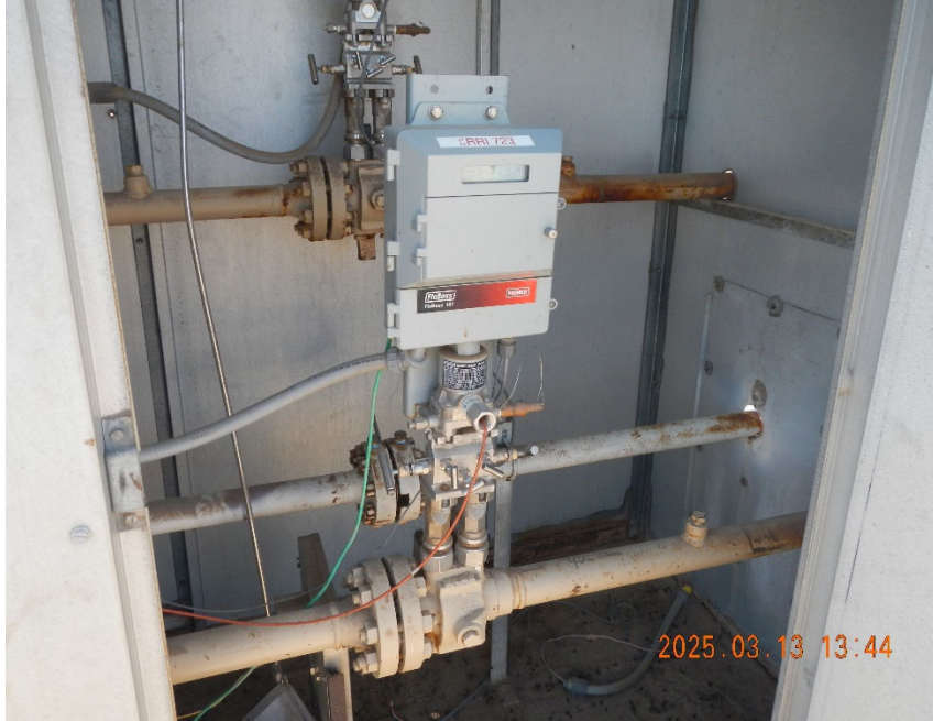
5. Gas meter inside meter shed.
