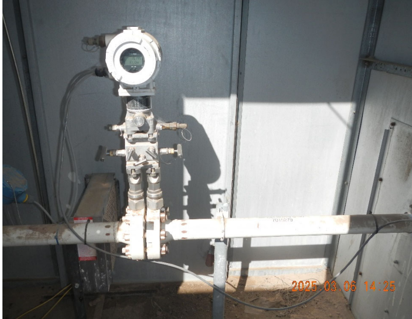
5. Gas meter inside meter shed.
