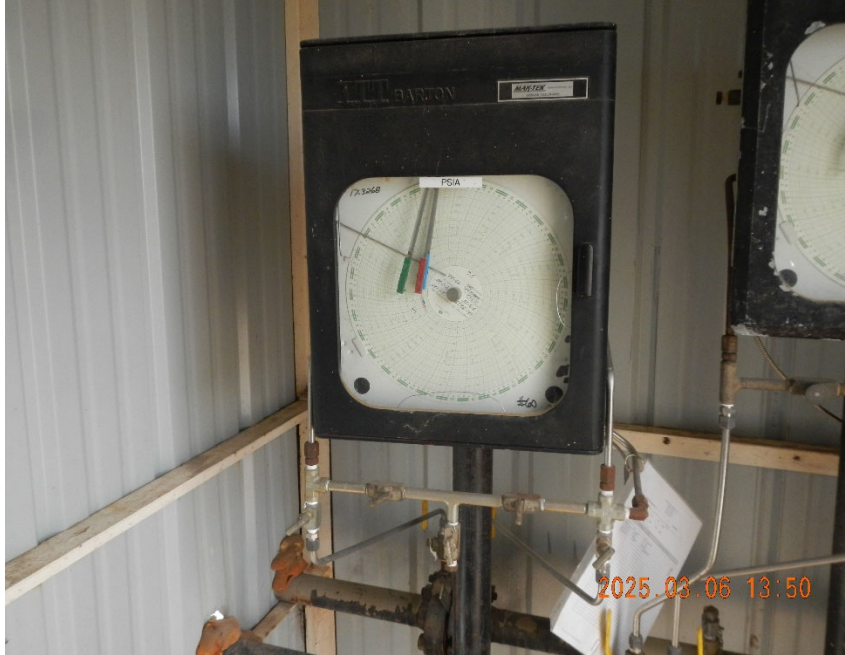
5. Gas meter inside meter shed.
