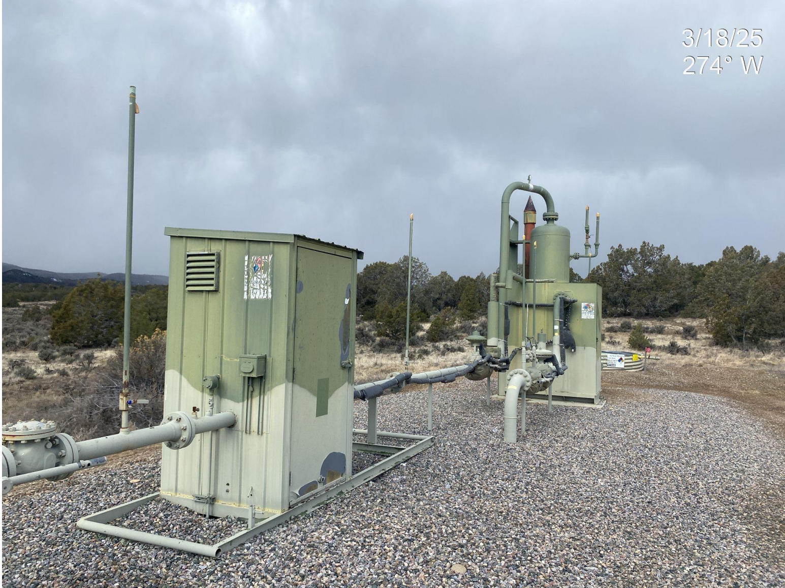
Photo 2. Labels at separator equipment has deteriorated and is no longer legible.
