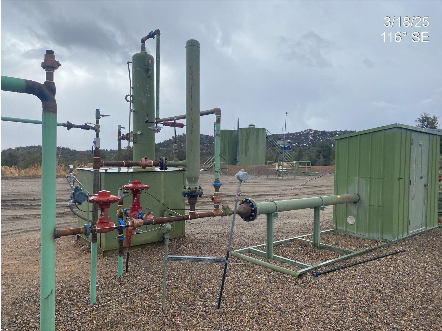
Photo 3. Unused equipment at separator equipment has been removed from location.
