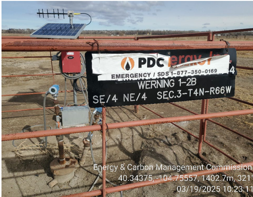
Wellhead and sign
