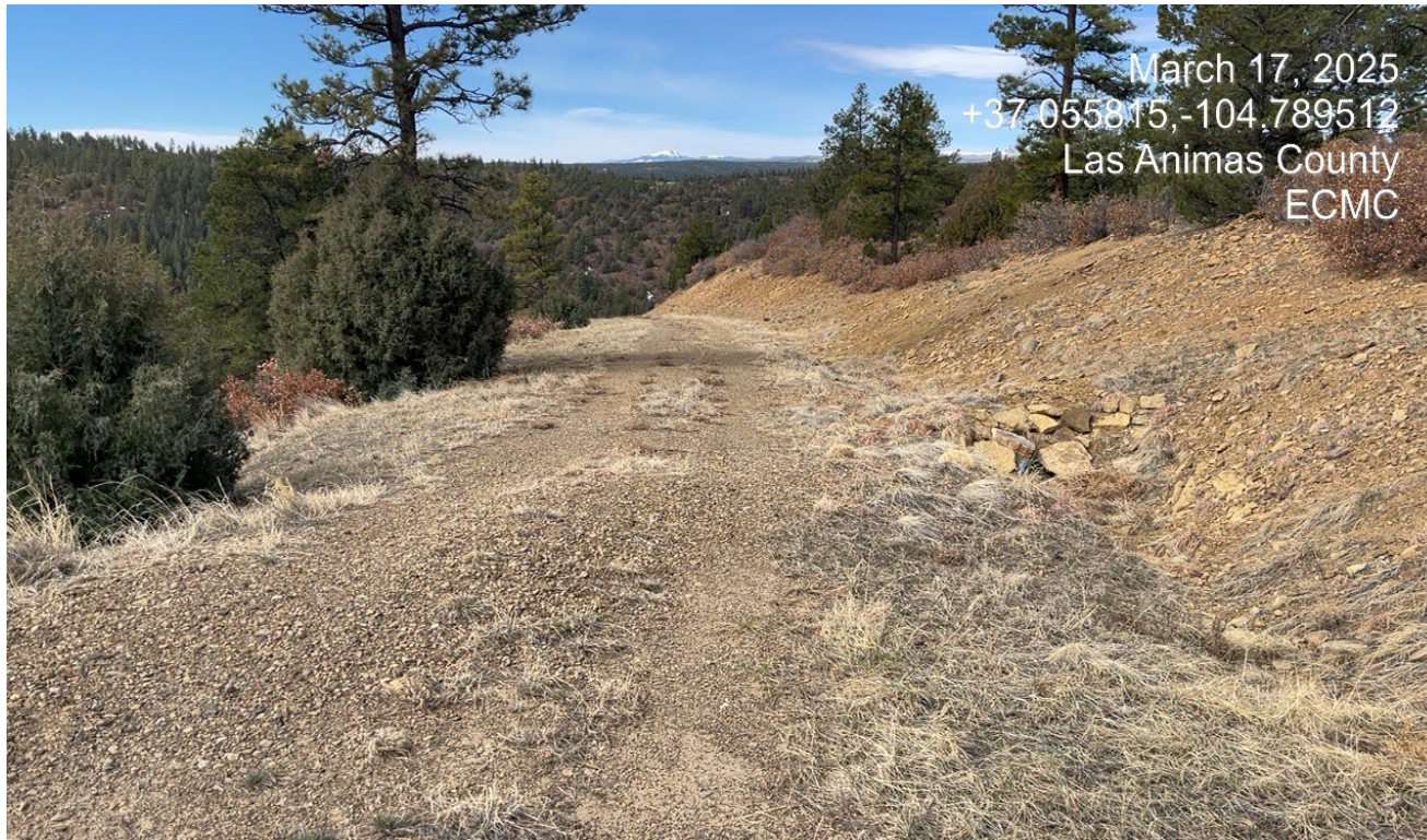
Photo 2. Facing southwest further along the access road. BMP's are installed and in good condition along the road.
