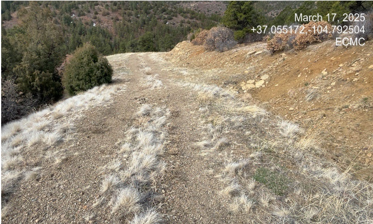
Photo 3. Facing south west further along the access road. BMP's are installed and in good condition along the road.
