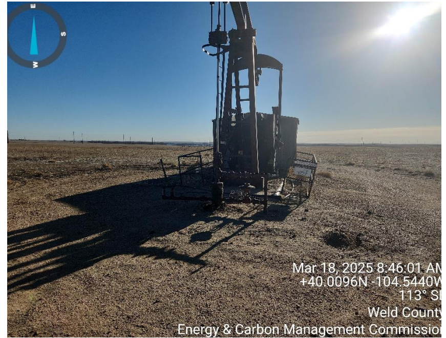
Photo 2 well head and equipment
