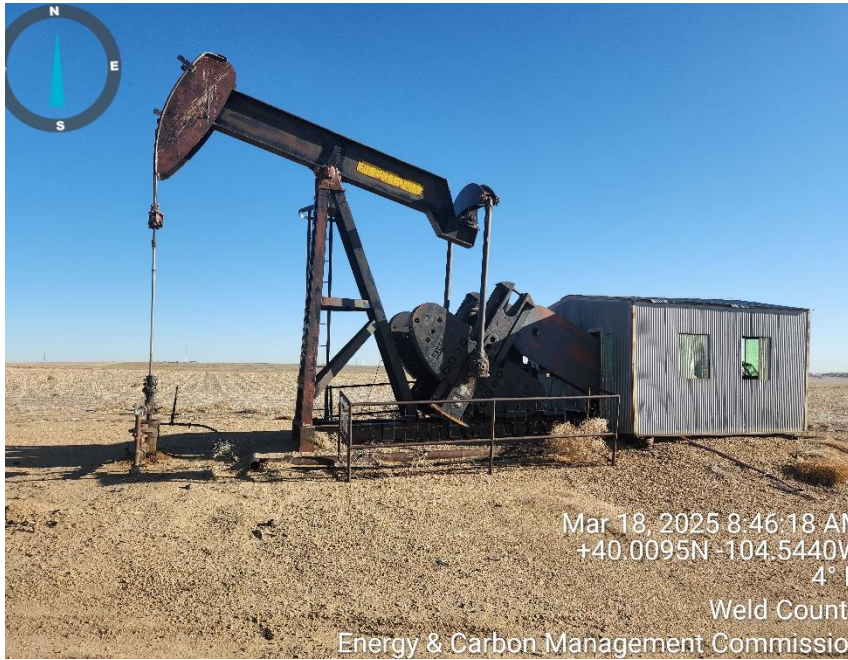
Photo 1 well head and equipment
