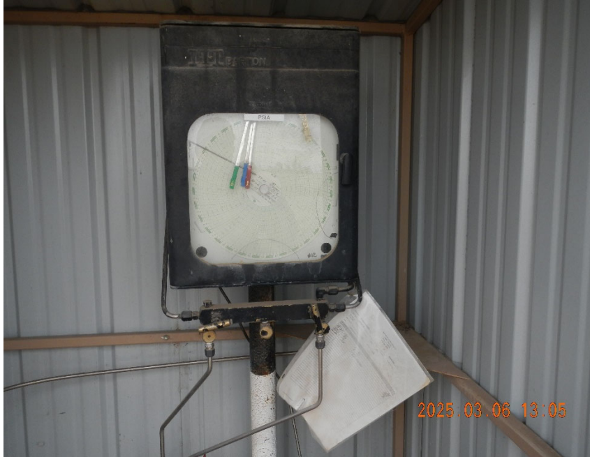
5. Gas meter inside meter shed.
