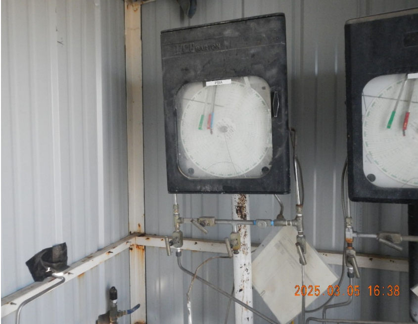
5. Gas meter inside meter shed.
