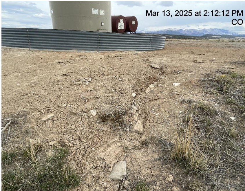
Photo # 3345 Erosion & transport of sediment off location /insufficient BMP's
