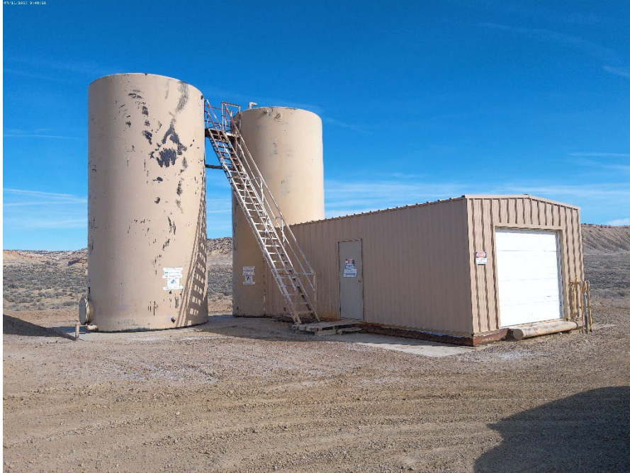
Pump housing and Tank battery
