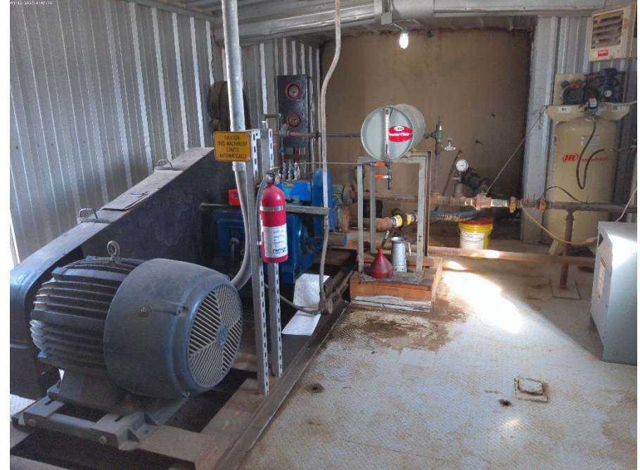
Injection pump inside housing
