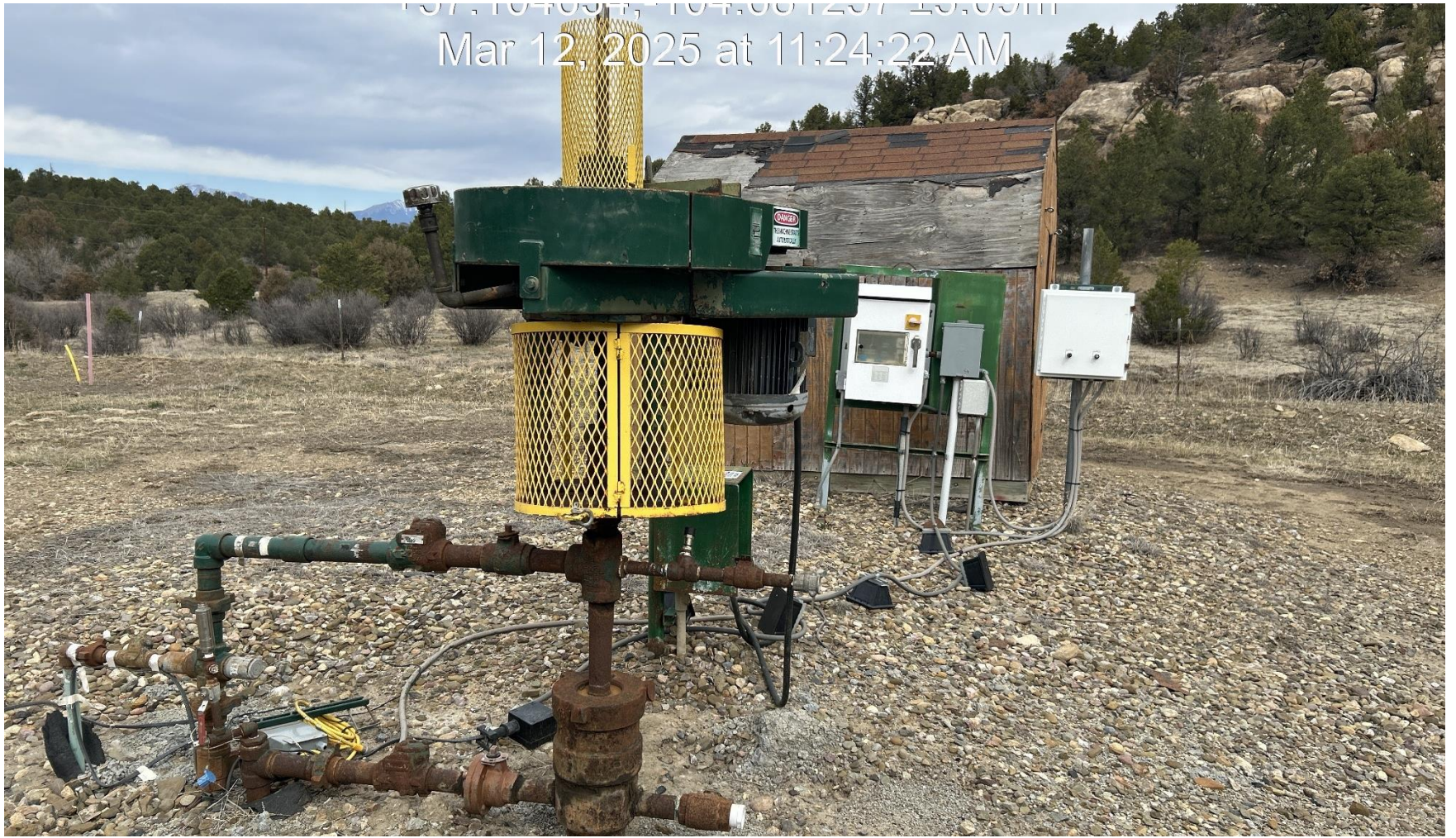
PHOTO 3: WELLHEAD AND EQUIPMENT
