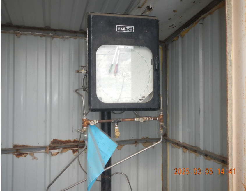
5. Gas meter inside meter shed.
