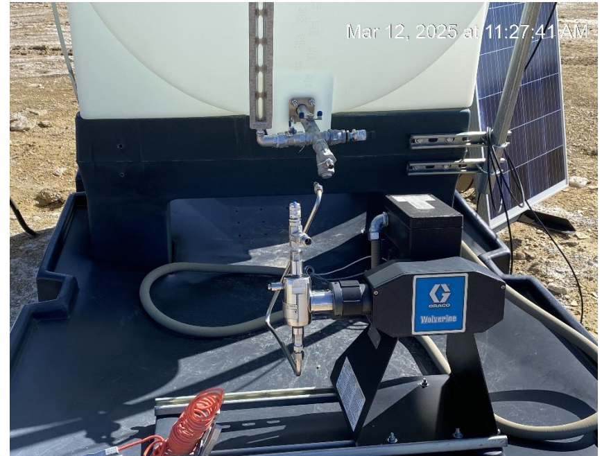
Equipment not in use
