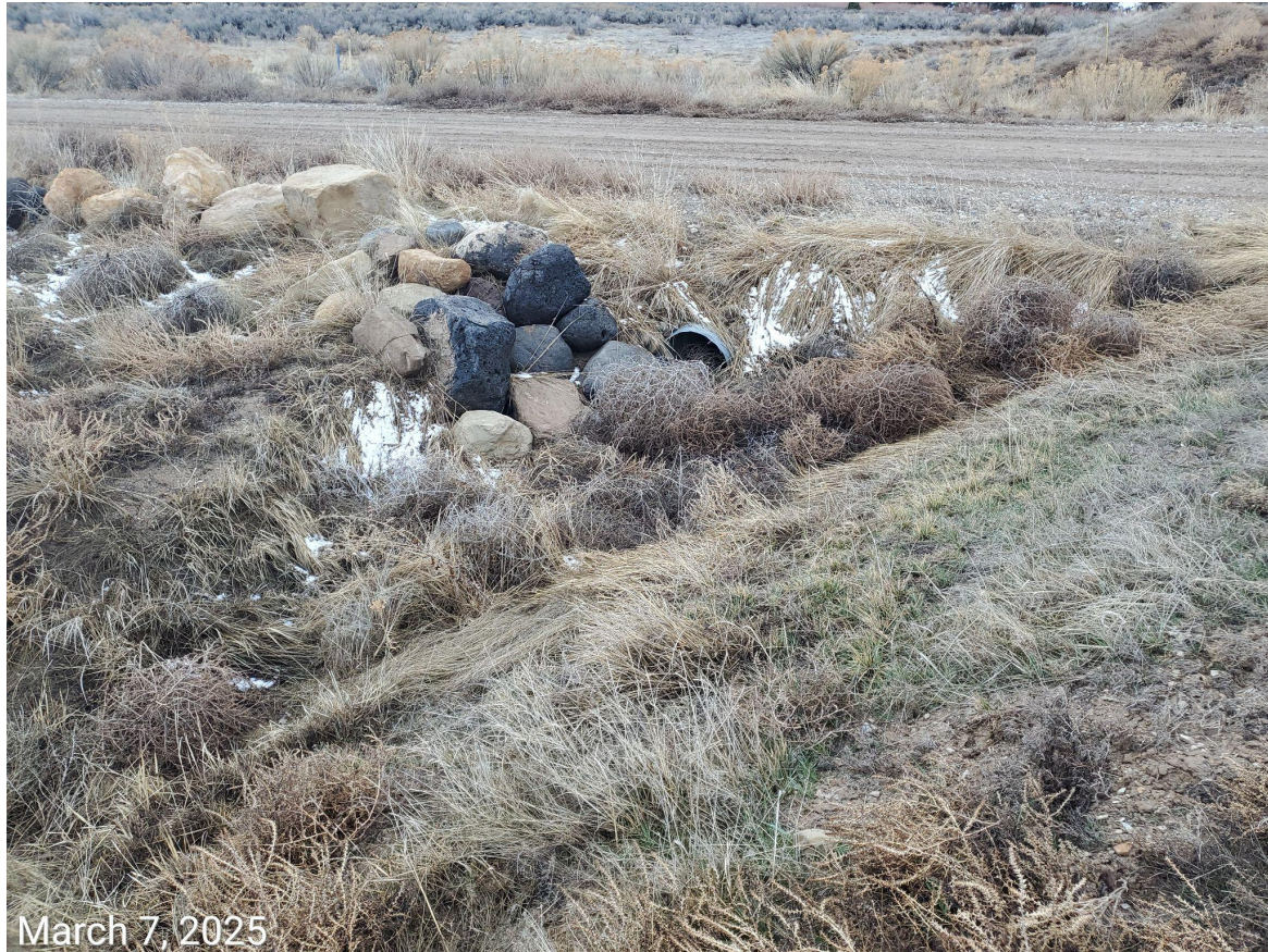
Photo 13: Photo taken from the east end of the Location, facing south. Photo shows weed debris accumulation within the ditch and culvert.
