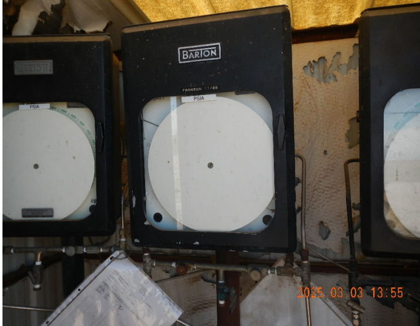
5. Gas meter inside meter shed.
