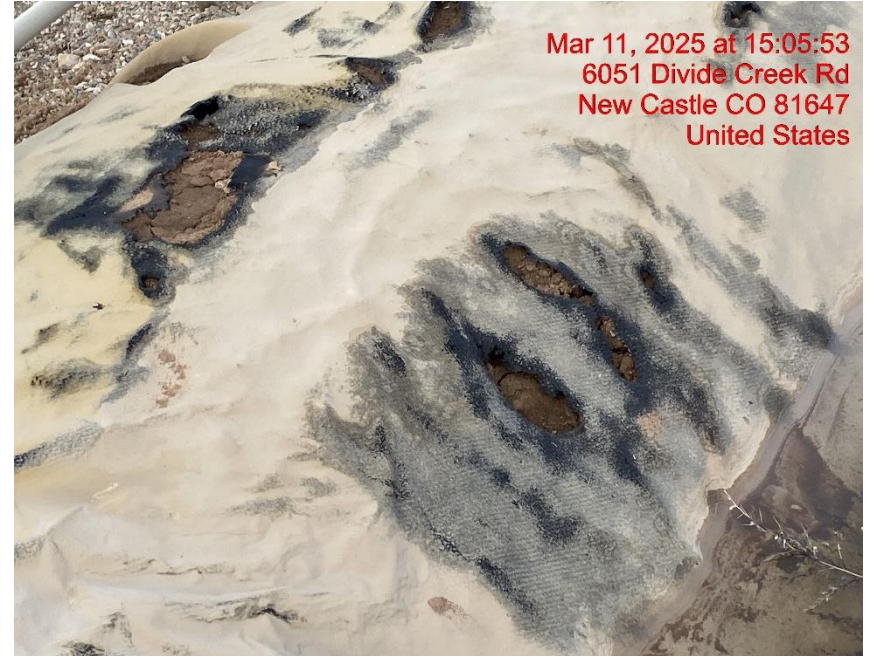
Unserviceable Berm Liner – Photo #07157
