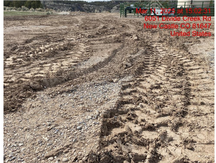
Lack of Stabilization – Photo #07151
