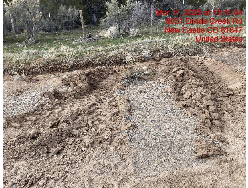
Lack of Stabilization/Degradation – Photo #07170
