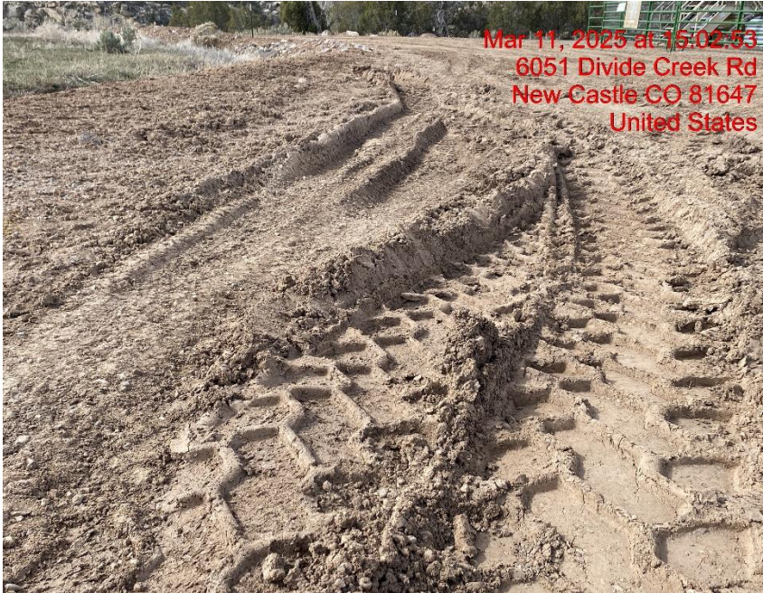
Lack of Stabilization – Photo #07152
