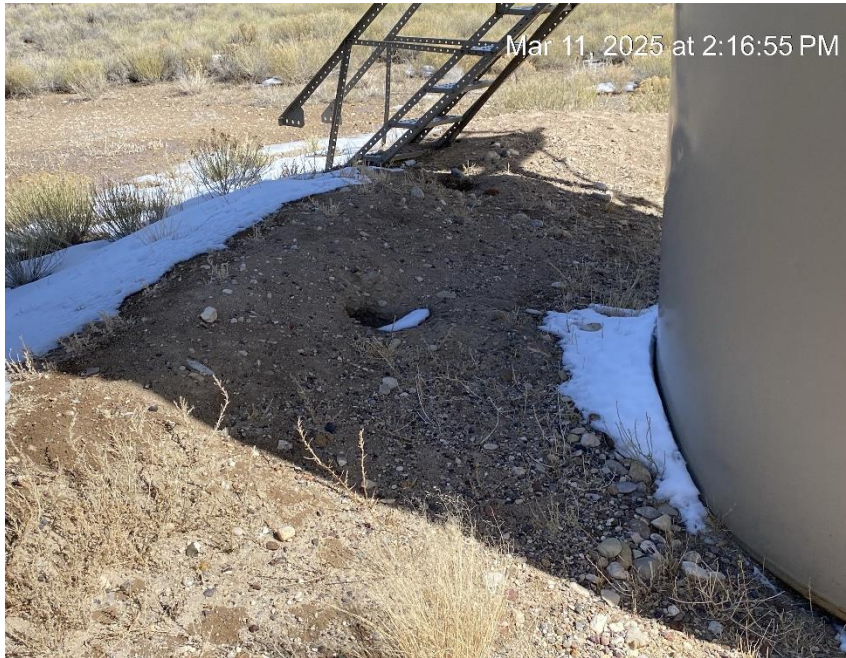
Berm capacity inadequate
