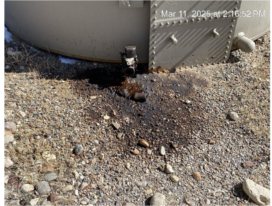
Open end tank valve. Spill.
