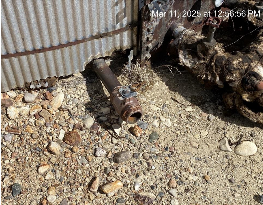
Open end tank valve
