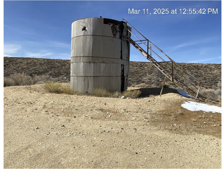
No sign at tank battery
