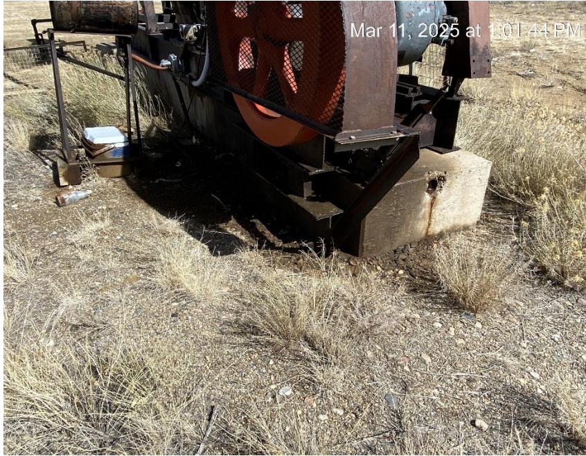
Oily waste and staining
