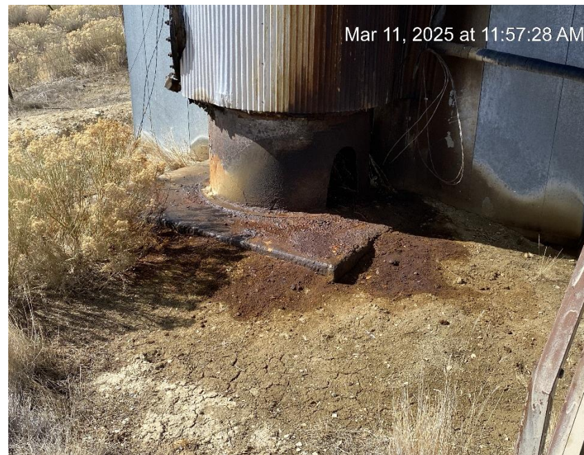
Oily waste and staining
