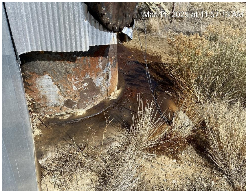
Oily waste and staining
