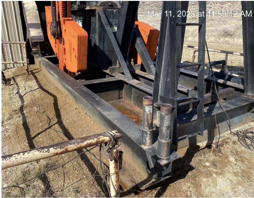
Debris. Oily waste and stained soil.
