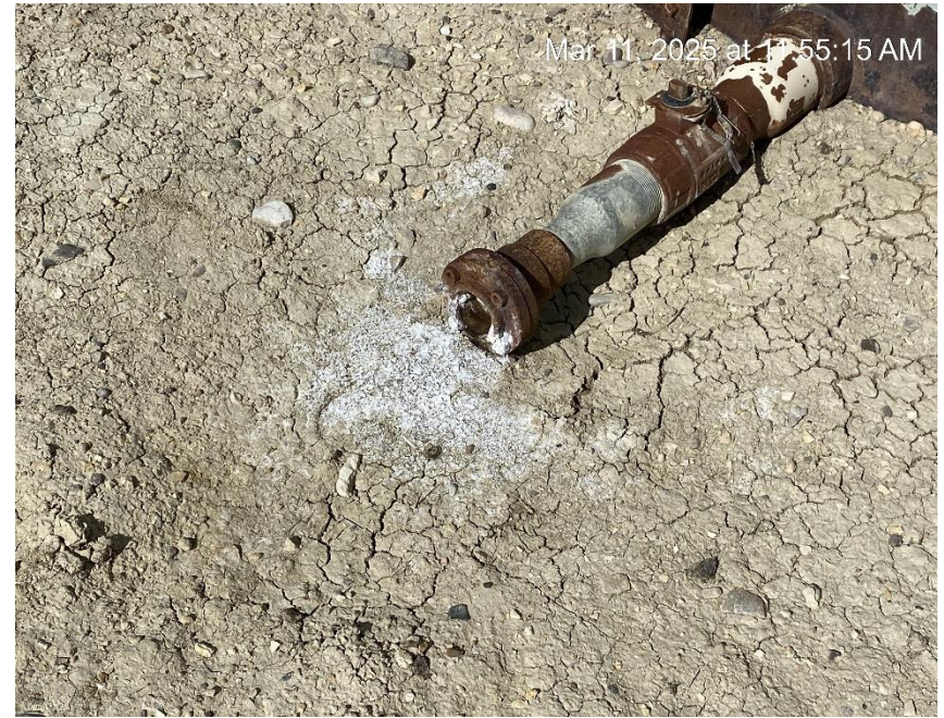
Leaking open end load line
