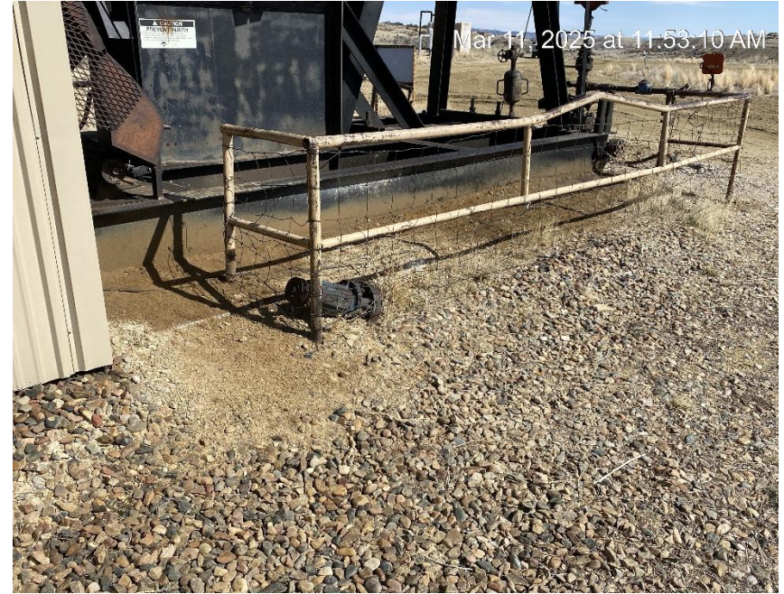
Debris. Stained soil.
