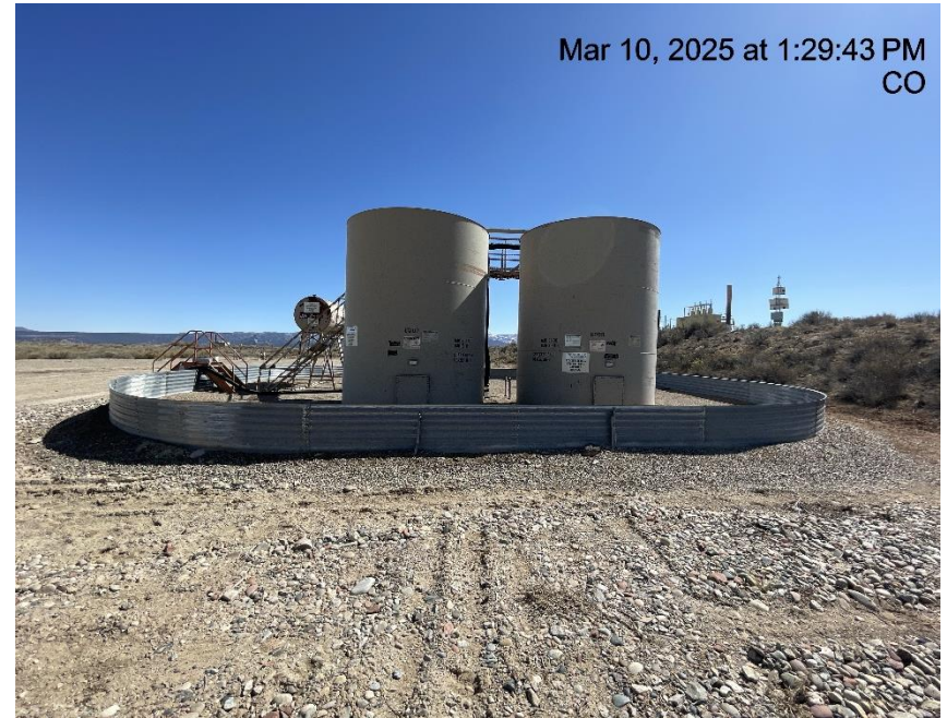
Photo # 1961 Battery lacks required signage
