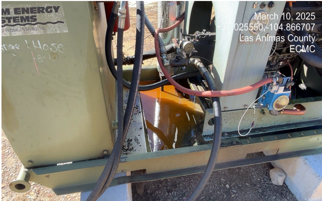
Photo 3. There is oily fluids in the engine skid that needs to be cleaned up.
