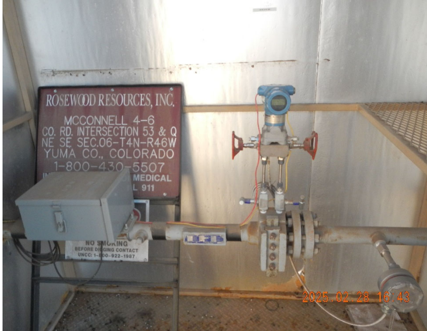
5. Gas meter inside meter shed.
