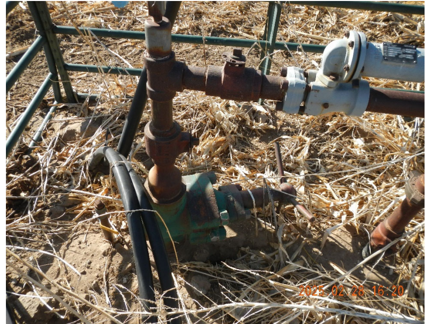
2. View of wellhead. Open ended black poly noted.
