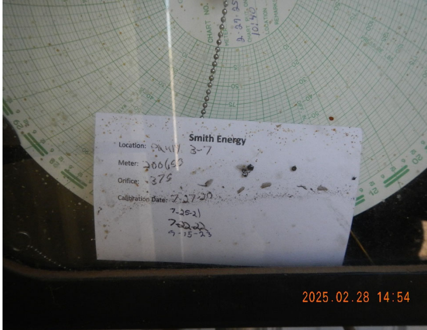
5. Meter calibration log inside meter box. Last calibration dated 9-15-23.
