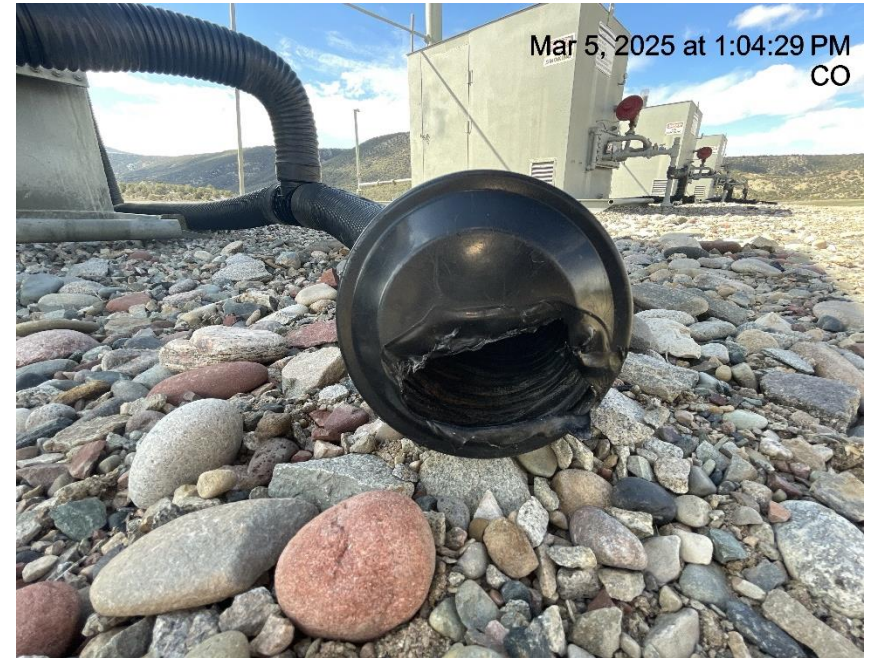
Photo # 819 Flowline heating insulation cap damaged /available for entry by wildlife/wildlife hazard
