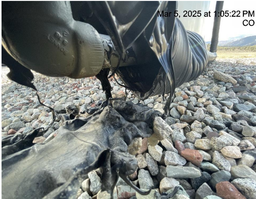
Photo # 820 Flowline heating insulation damaged/available for entry by wildlife/wildlife hazard
