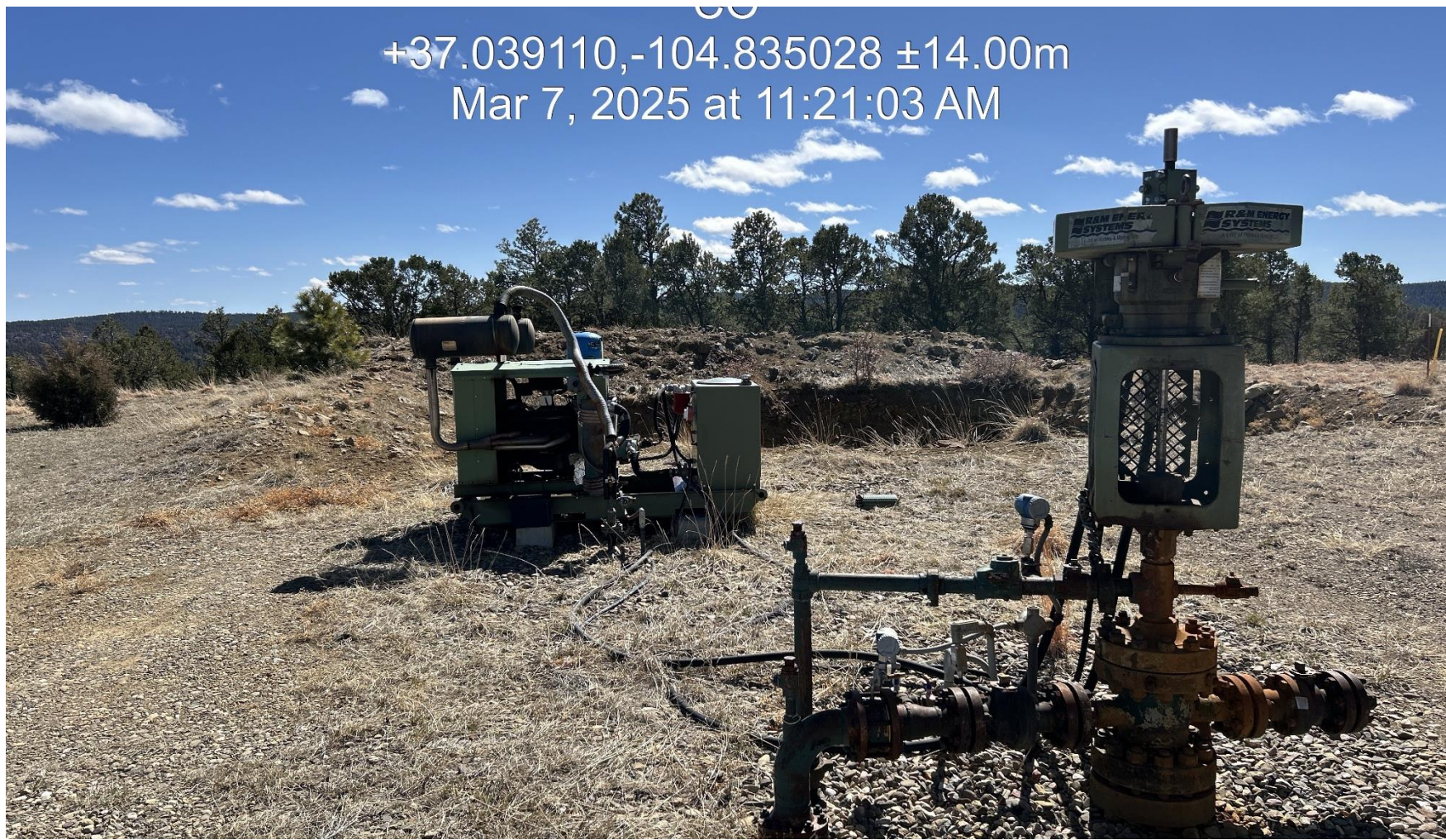
PHOTO 3: WELLHEAD AND EQUIPMENT
