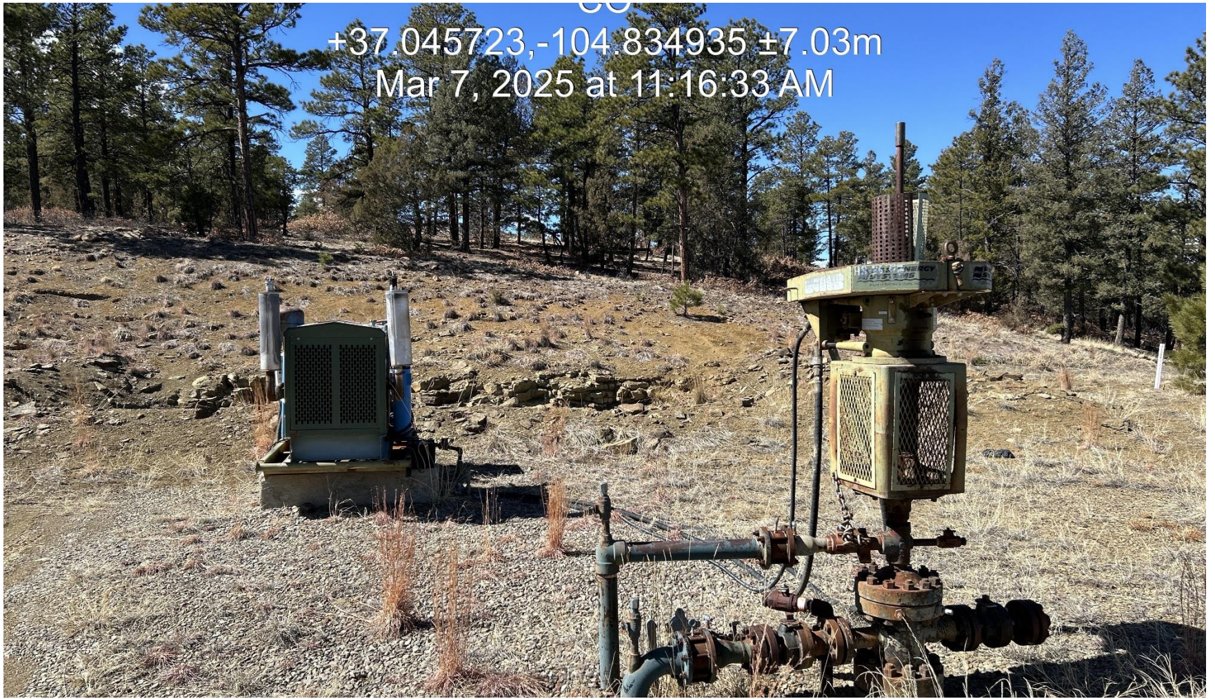
PHOTO 3: WELLHEAD AND EQUIPMENT
