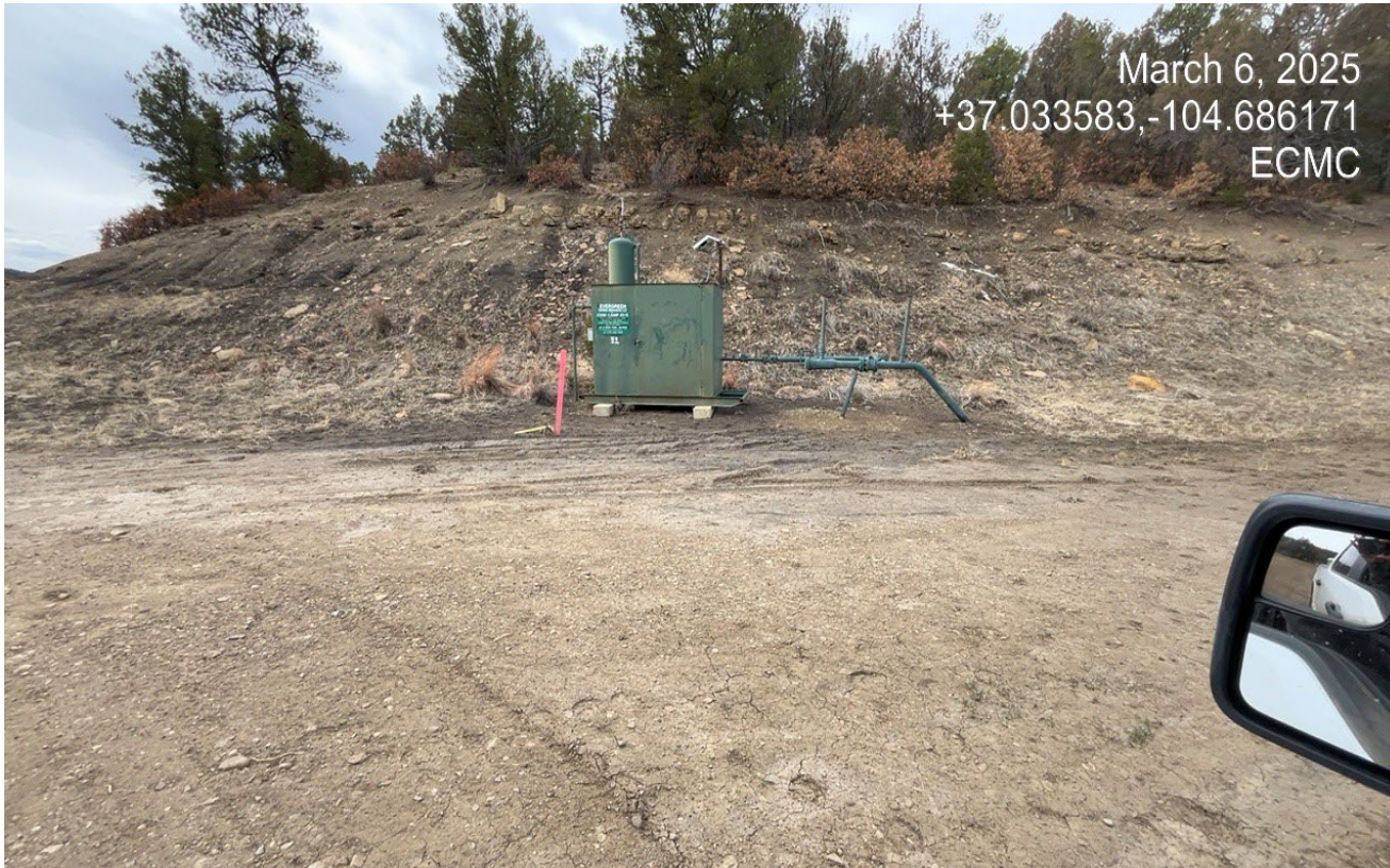
Photo 3. Well sign is posted at the meter shed.
