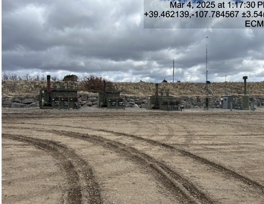
Location/ lack of stabilization
