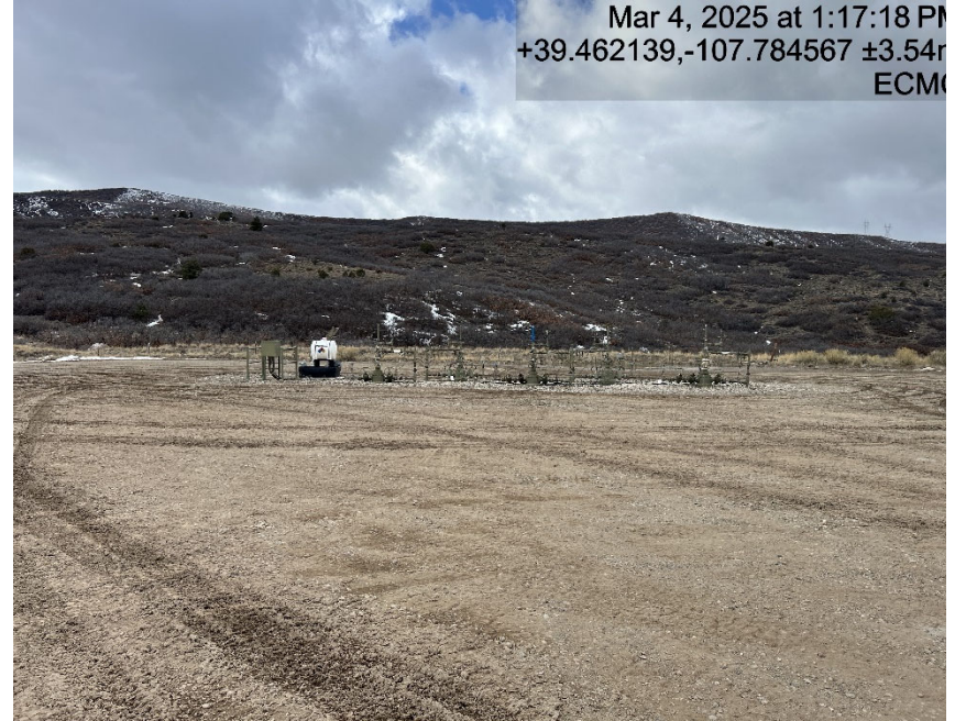
Location/ lack of stabilization
