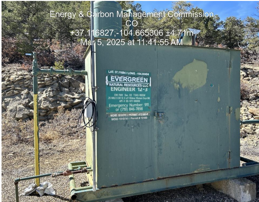
Photo 3 Meter house & well sign
