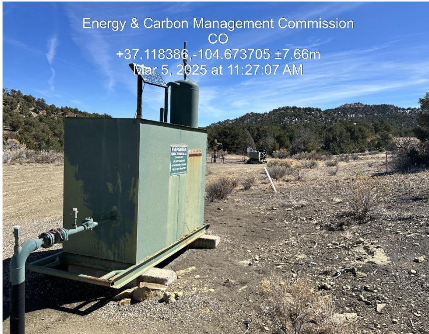
Photo 3 Meter house & Well sign
