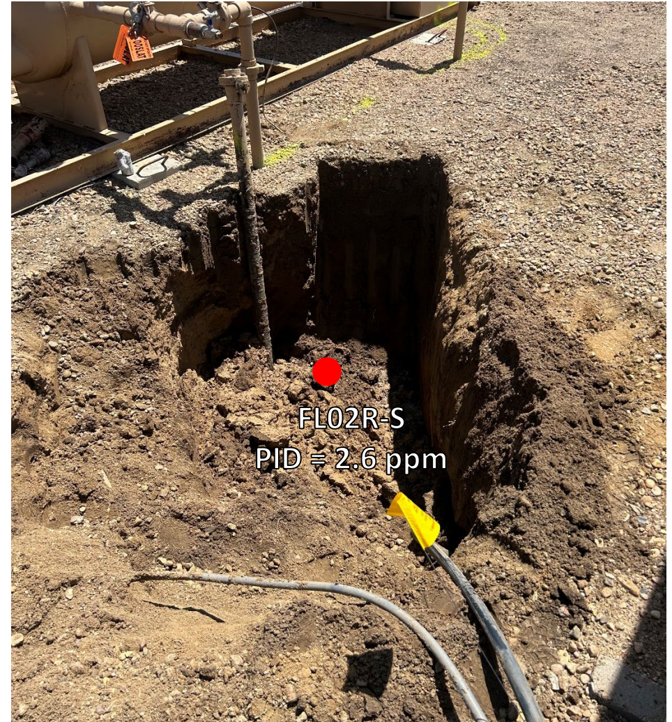
Looking south at flowline Pt B/terminus at separator No petroleum hydrocarbon staining or odor observed
