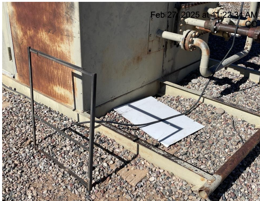
Photo # 9955 Wellhead sign laying on ground near separator/sign not properly posted
