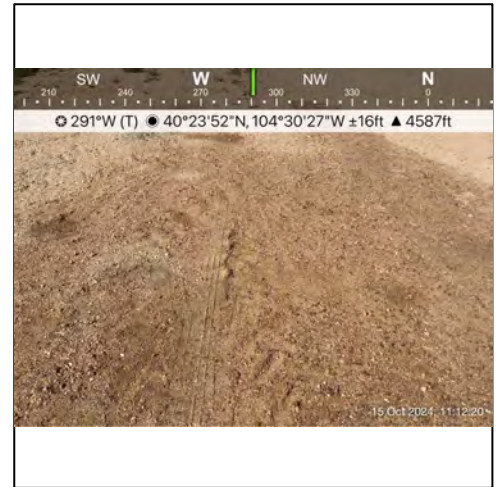
P6 - Clean road base and backfill have been employed to match the existing contour.
