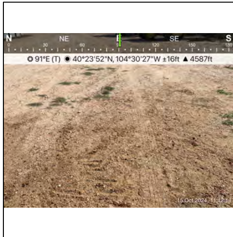
P5 - Clean road base and backfill have been employed to match the existing contour.
