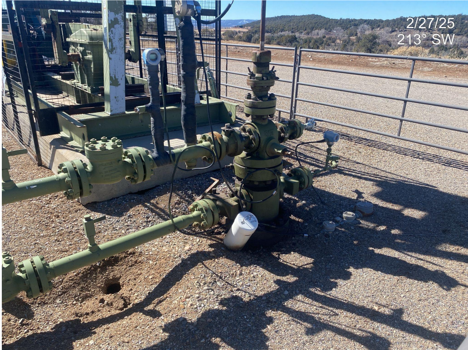
Photo 3. Stained soils at the wellhead have been removed/remediated.
