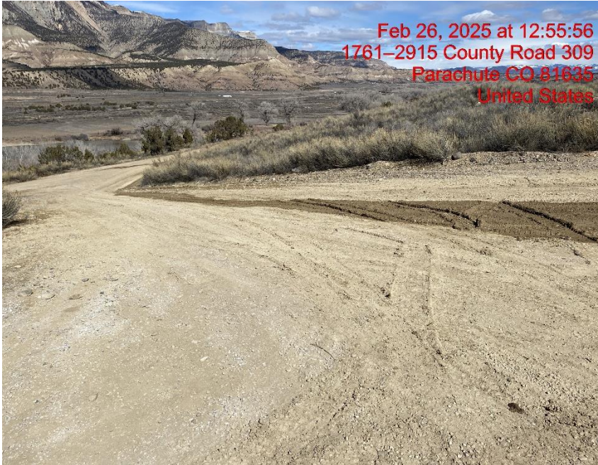
Insufficient Tracking BMPs – Photo #06892
