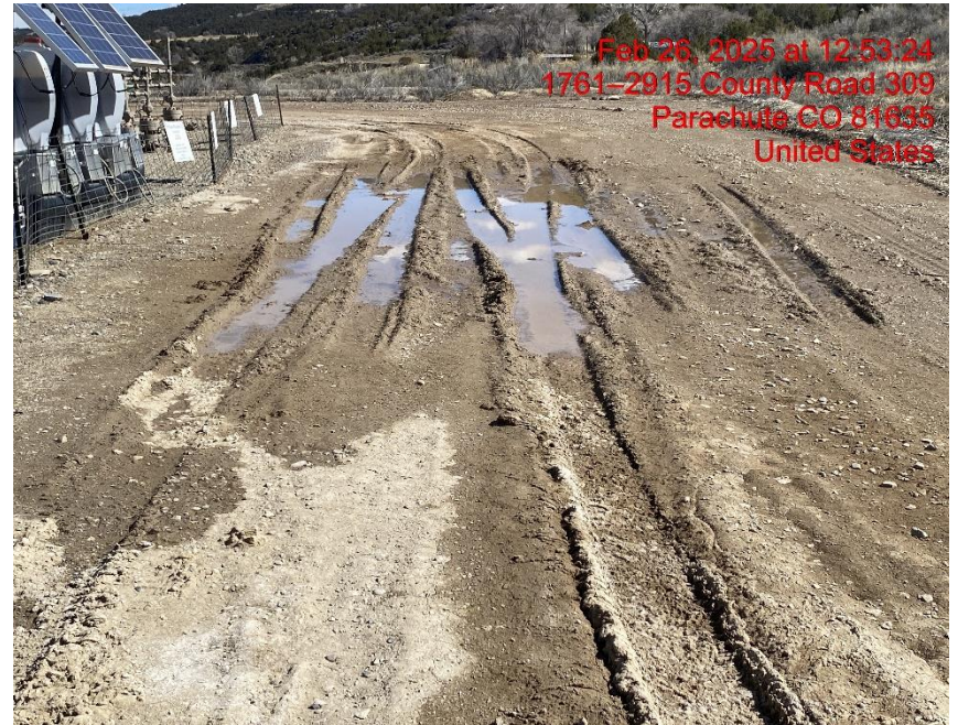
Lack of Stabilization – Photo #06887
