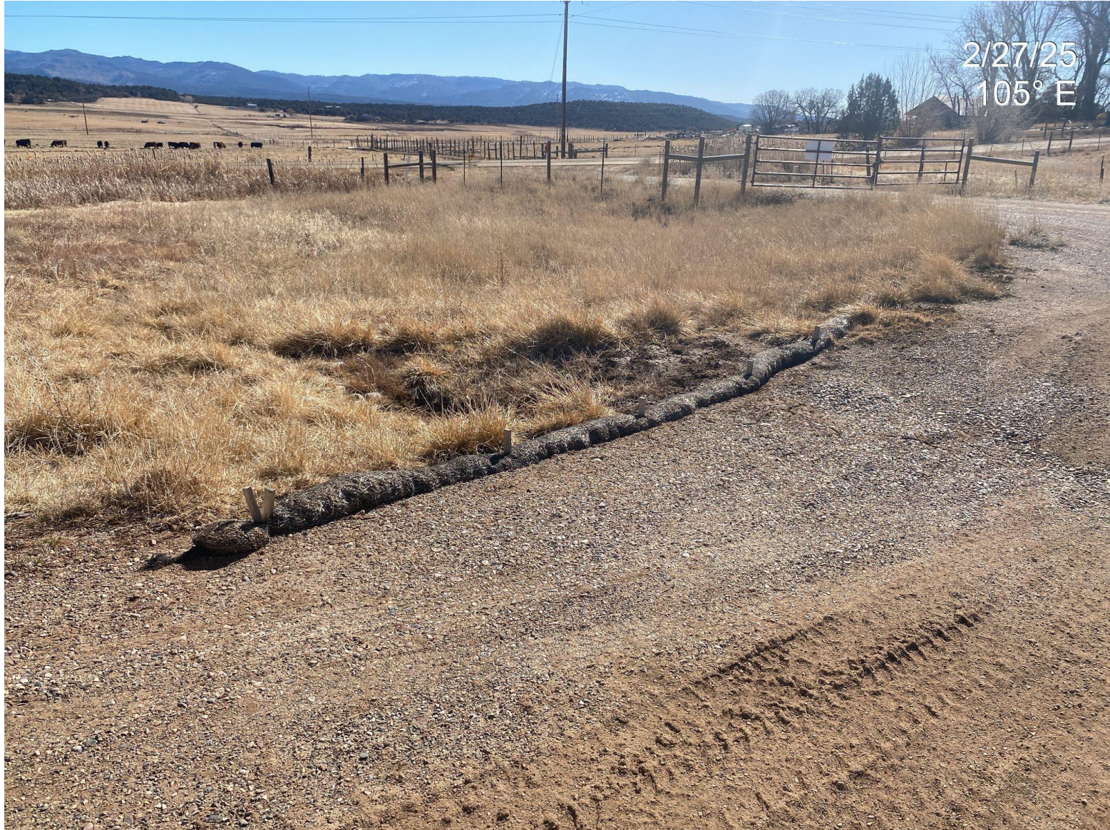
Photo 3. Stormwater BMPs installed in the eastern portion of the pad.
