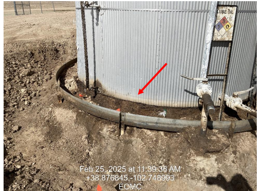
Photo 10 – Impacted soils present under tank
