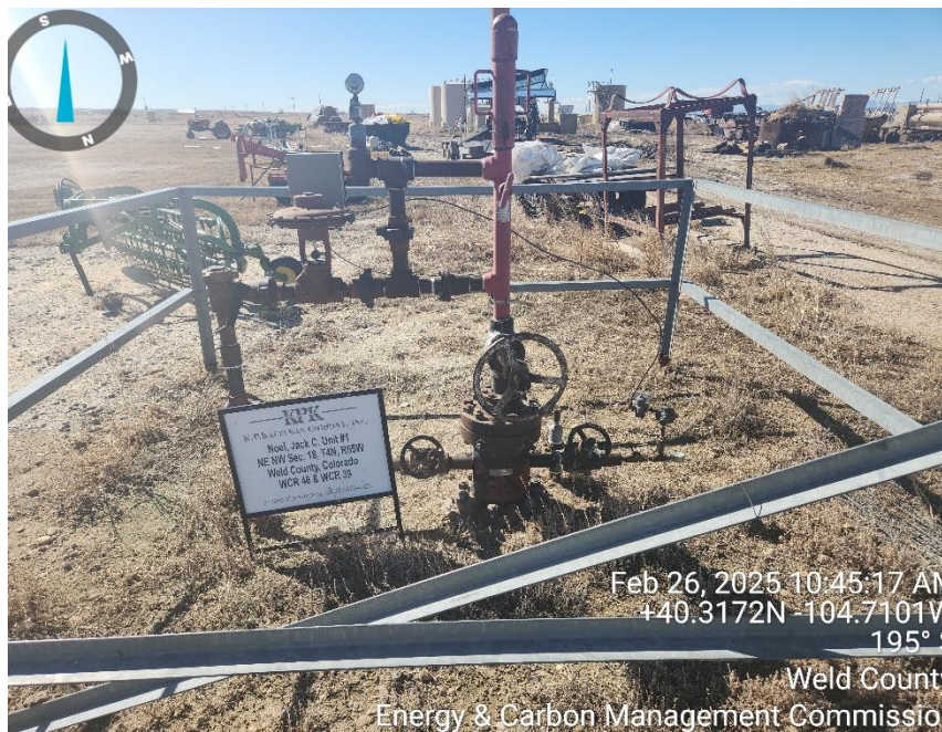
Photo 1 well head and equipment
