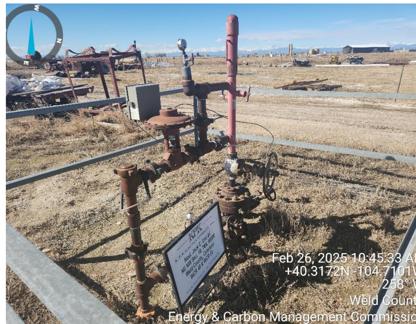
Photo 2 well head and equipment
