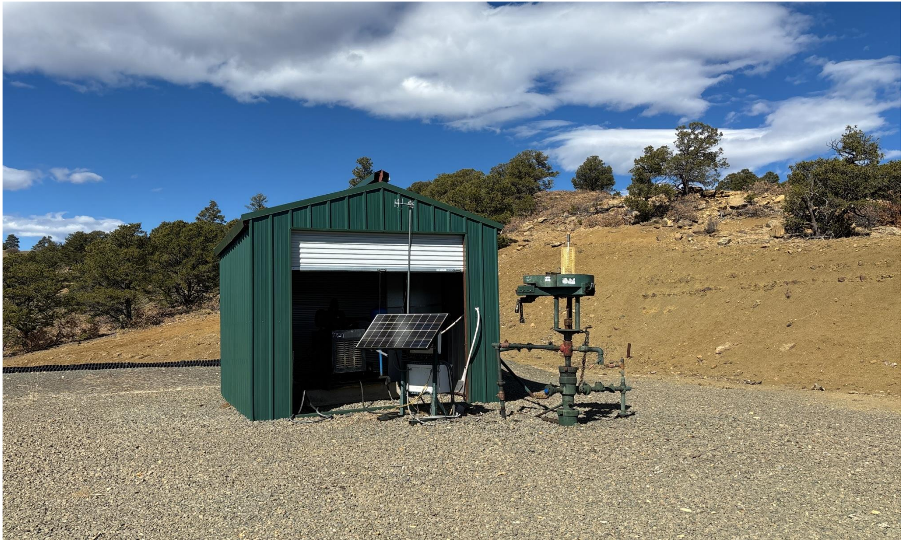
PHOTO 3: WELLHEAD AND EQUIPMENT.
