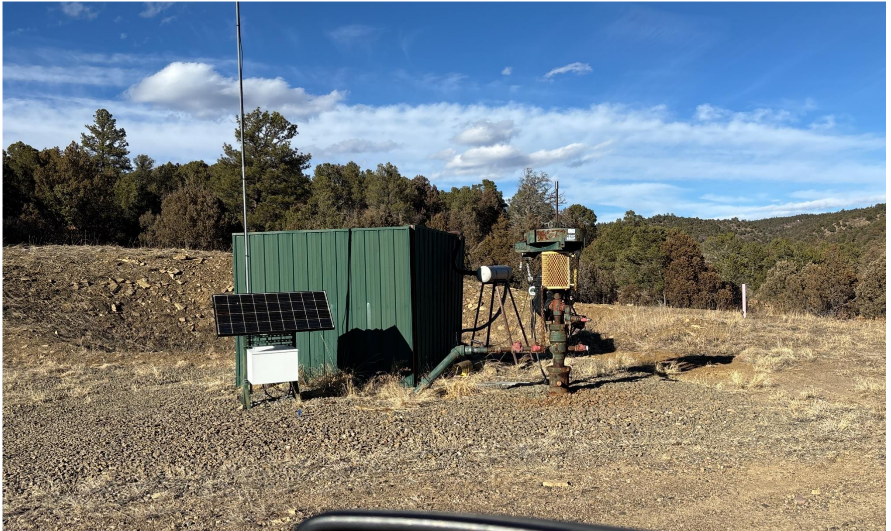
PHOTO 3: WELLHEAD AND EQUIPMENT.
